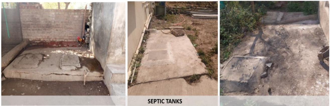
Figure 15 Septic Tank (Rural)
