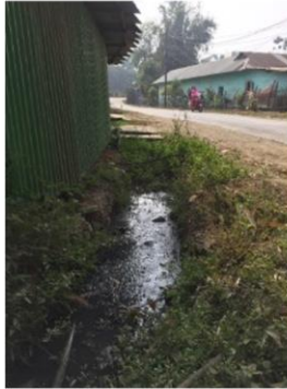
Unlined, open drains
